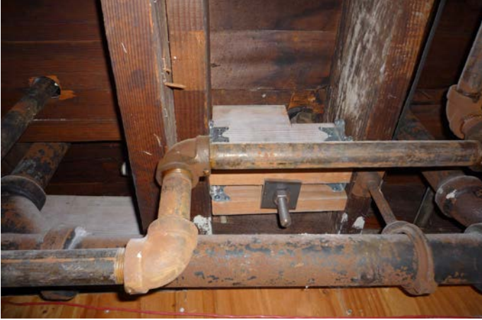
Rust and corrosion on pipes.
