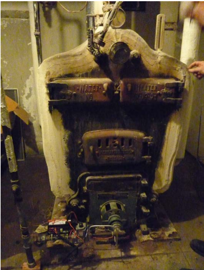
Original water heater.
