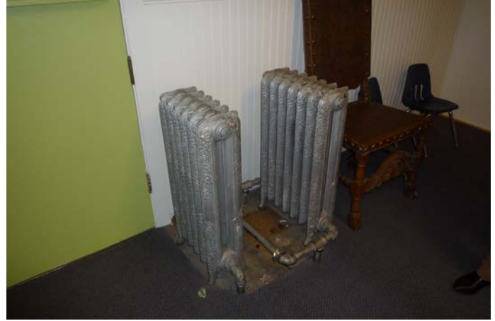
Asbestos composition tiles at radiator at pool table room, second floor.
