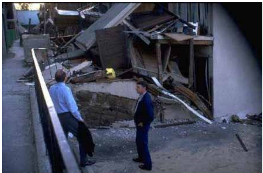
Roof Collapse Porches and balconies can collapse if not properly attached.
