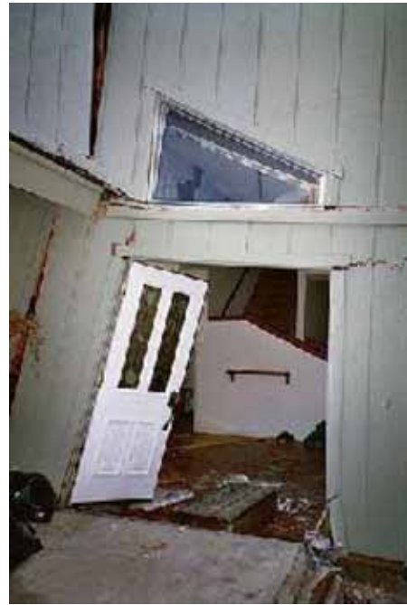
Unbraced cripple walls collapse.
