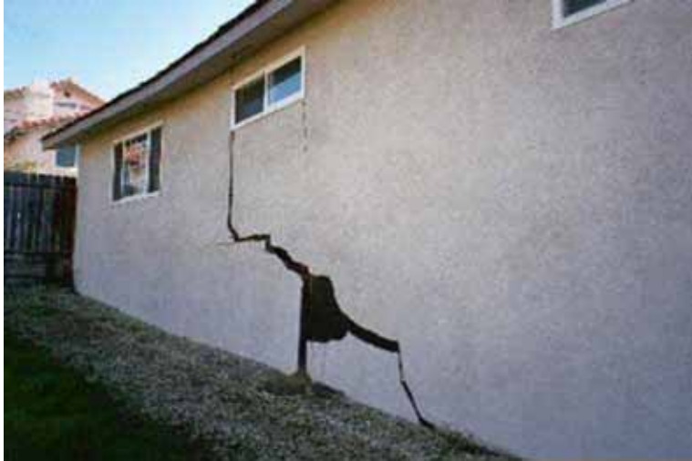
Houses that aren't bolted to their foundations shift off them.
