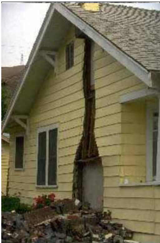
Chimney collapse is a widespread problem.
